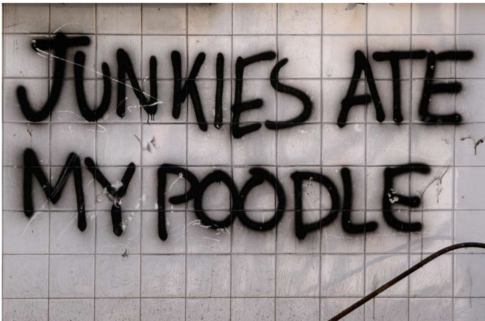
Graffiti at Ravelrig House prior to restoration
